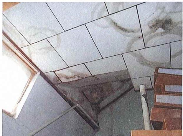
Suspect mold garage 2
