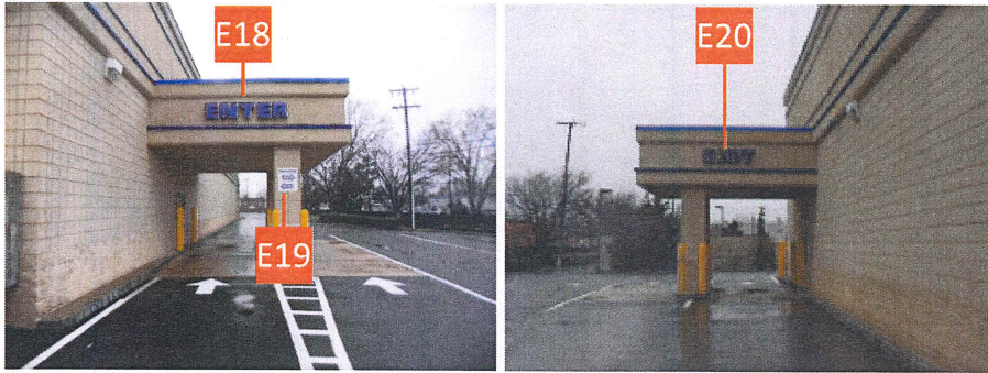
Existing signs to be removed; wall to be patched and painted as required
