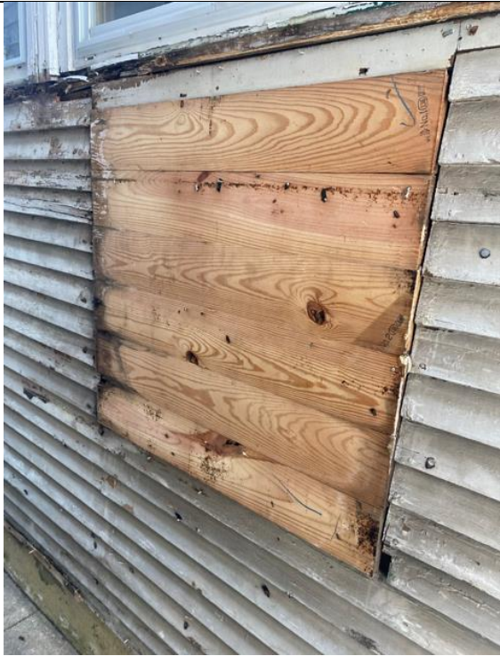
7: recent wood patch where window size was modified. Rot/siding damage
