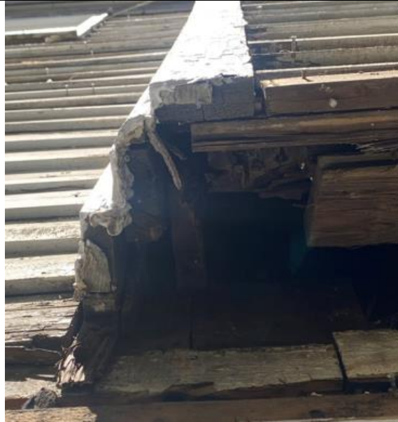
14: severe deterioration and rot of elements around area. daylighting is occurring at bottom of projection.
