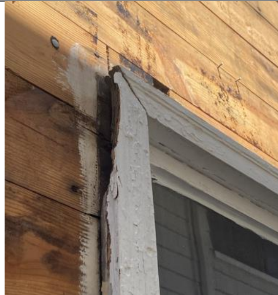
4: cracked, deteriorating window trim. Not original.
