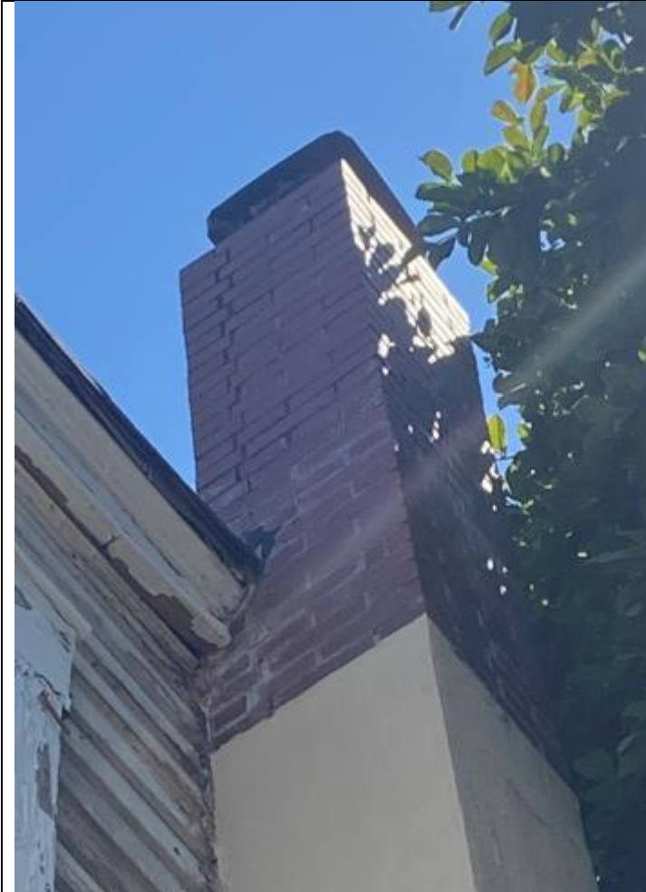
15: Exposed brick at top of rear (non-historic) chimney in poor condition
