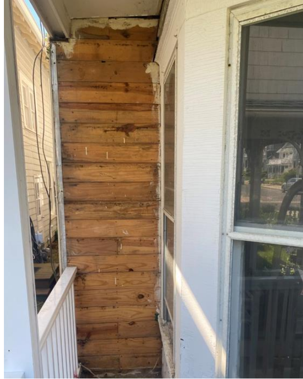
6: Evidence supporting the porch was enclosed as an addition. There was no siding behind the removed asbestos shingles.
