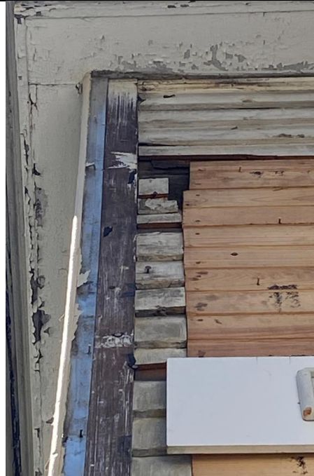
8: Clapboard around patch on rear second floor projection appears to match primary material used throughout the structure but has been damaged and cracked over the course of the structures history.
