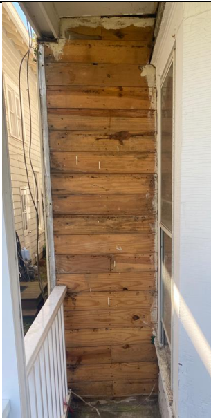
13: sheathing boards indicate areas of porch that were enclosed at a later date and are not original of the historic structure
