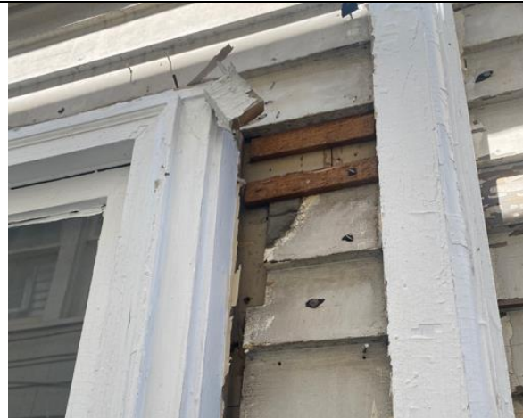
8: clapboard is cut, cracked, and missing. clapboard shows evidence of original window trim profile. Current trim is deteriorating and broken, most likely designed after asbestos siding installation.
