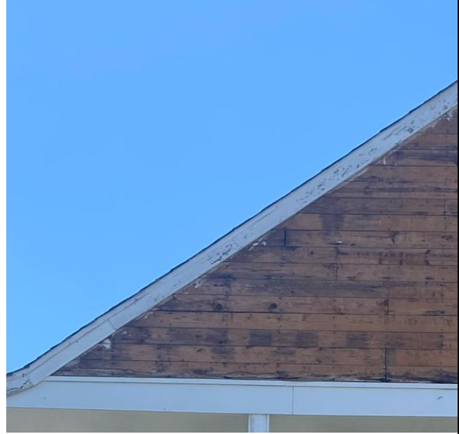
12: wood sheathing boards at gable end of porch roof indicate this roof was added at a later date and was not original to historic structure
