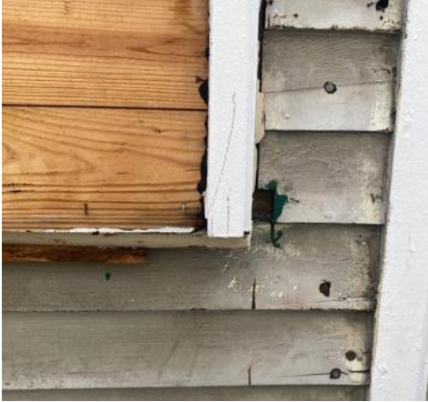
9: sill profile not present, original opening most likely patched and trim designed to accommodate asbestos siding.
