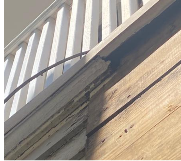
1: trim and clapboard cut haphazardly to meet wood sheathing infill
