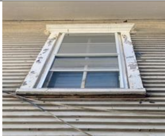
2: window casings in poor/fair condition. Rot at underside of sill indicates signs of water infiltration.
