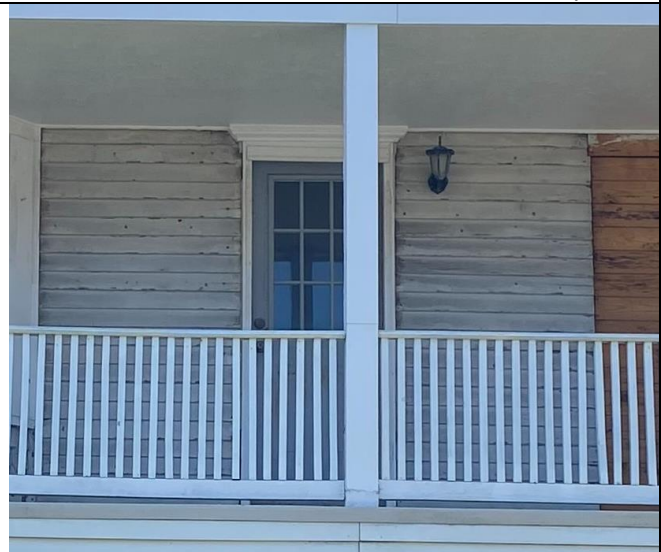
10: 4" Exposure Wood Clapboard in fair condition below porch but many nailholes, rot around edge boards, and large patched areas where windows/doors were relocated
