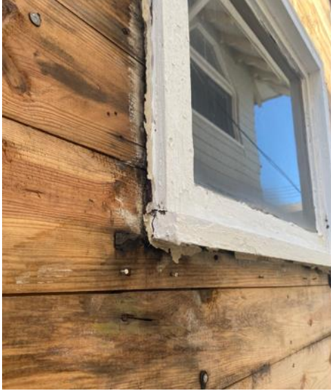
5: Windows in additions (newer wood sheathing) are in poor condition as well
