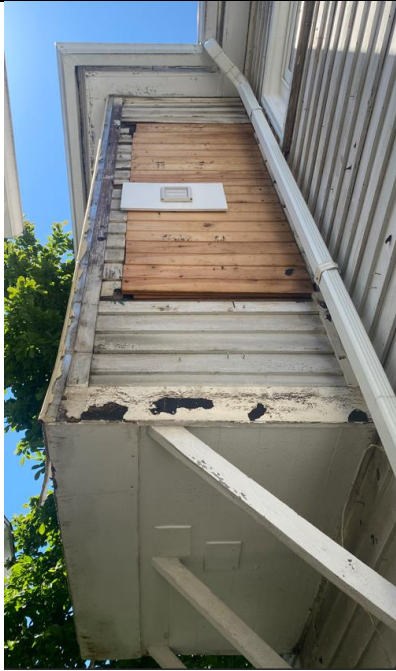
7: Patchwork with tongue and groove boards completed on rear second floor projection.
