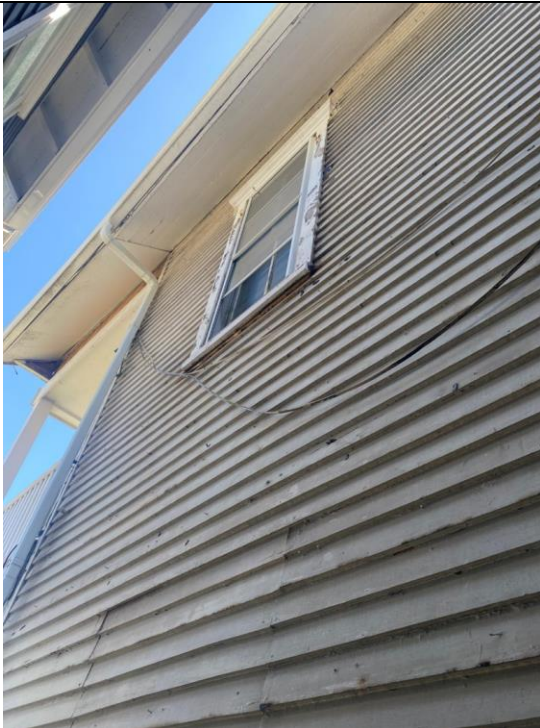
17: Siding in poor condition. Excessively nailed, patched, and cracked
