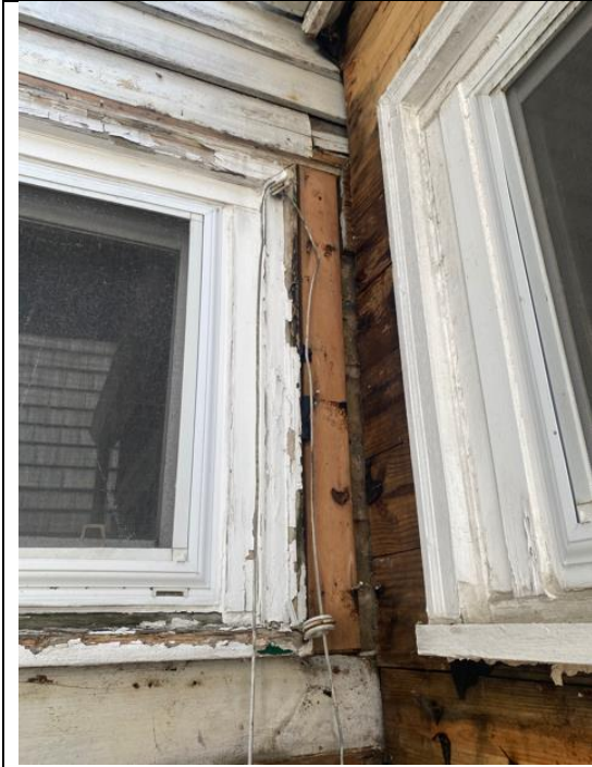
11: excessive rot/patchwork and infill of openings
