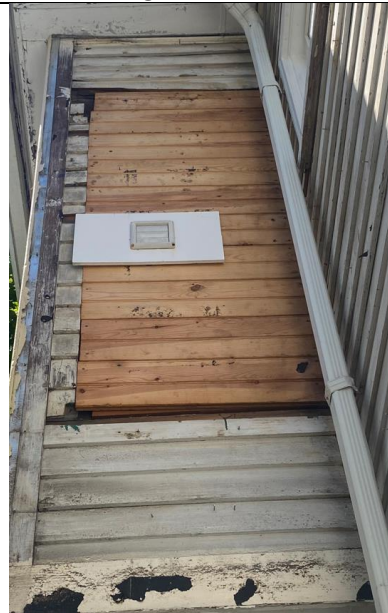
14: siding cut/in poor condition
