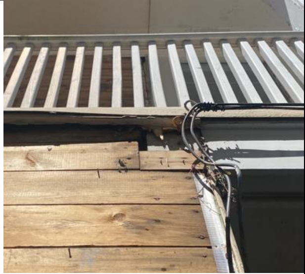
2: haphazard patching of sheathing boards with large gaps between siding/sheathing
