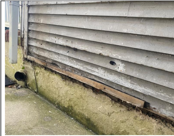
1: rot/deterioration at base. Excessive nail holes. Rot at corners.
