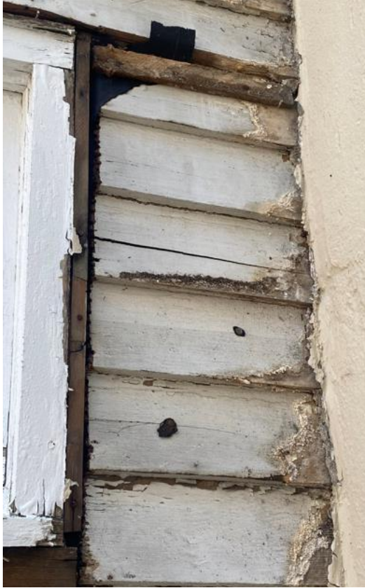
5: cracked, rotted, and deteriorating siding between window opening and stucco chimney.
