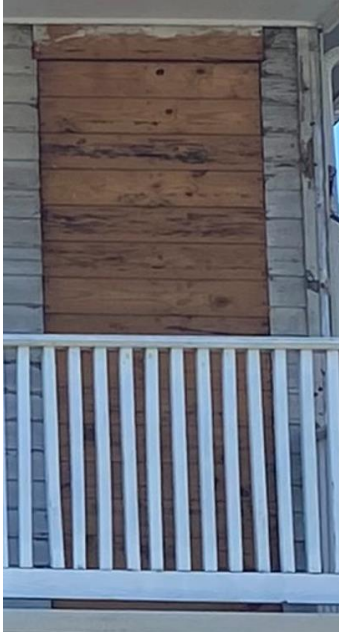
11: window/door openings patched with wood sheathing boards
