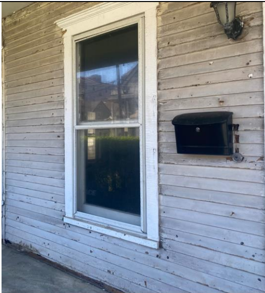
9: 3" Exposure Wood Clapboard in fair condition below porch. Damaged boards around edges and many nail holes from "layering" of siding
