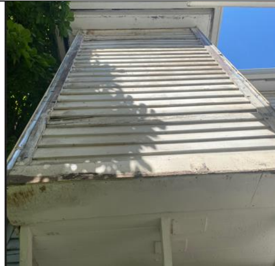
16: severe deterioration and rot at bottom of projection creating a daylighting condition.
