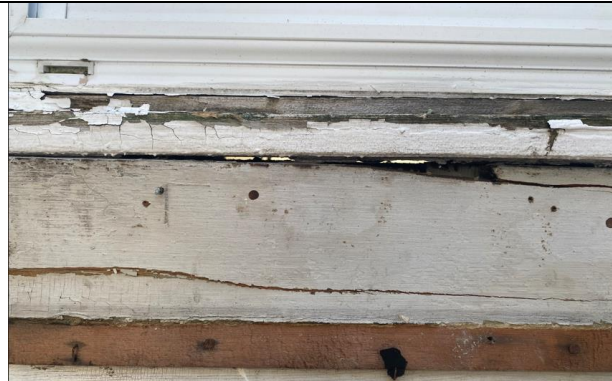
10: significant rot/deterioration at door casing and siding.
