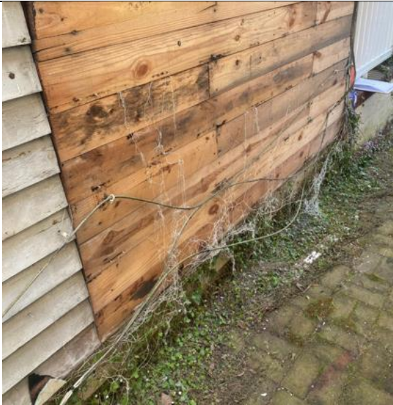
3: wood clapboard cut and patched. Excessive nailing. Rot evident at lowest courses and around windows/doors.
