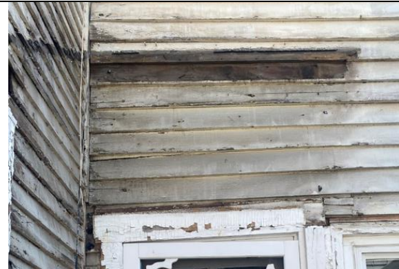
9: significant rot/deterioration at door casing and siding.
