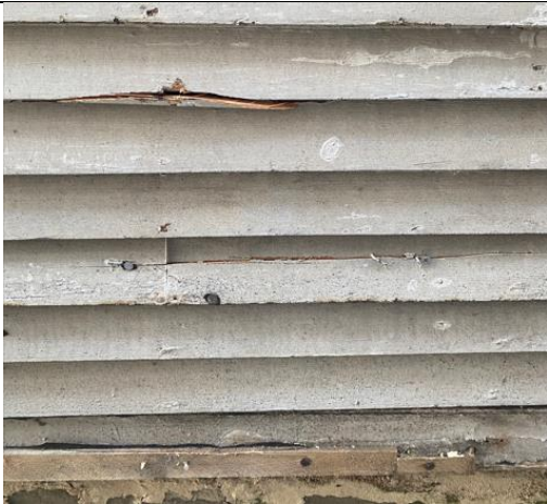
3: Cracked boards throughout
