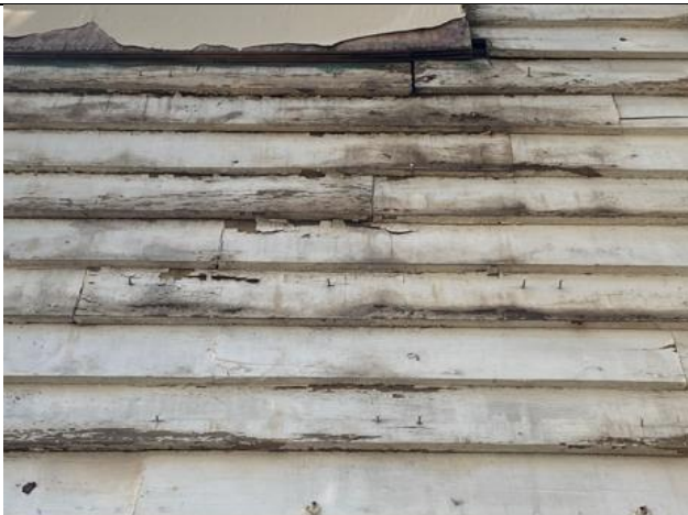
17: siding in poor condition, excessively nailed, patched, and cracked.
