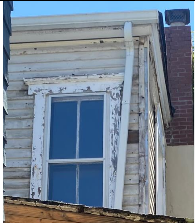
18: Siding in poor condition. Excessively nailed, patched, and cracked. Window casings improperly installed, likely poor repair work.
