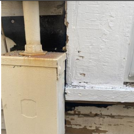
7: Siding/trim is cut/notched around exterior utilities.
