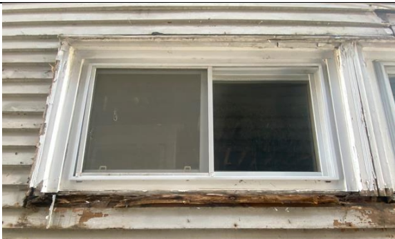
5: significant window frame rot
