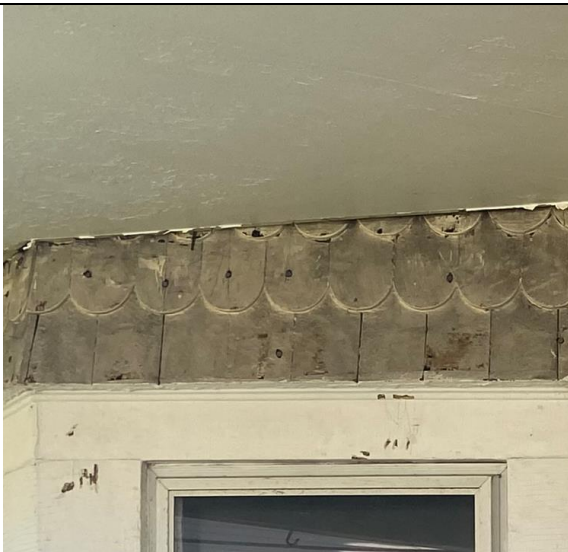
3: Evidence that the porch was added to the structure later because the scalloped shingles continue through the porch ceiling plane.
