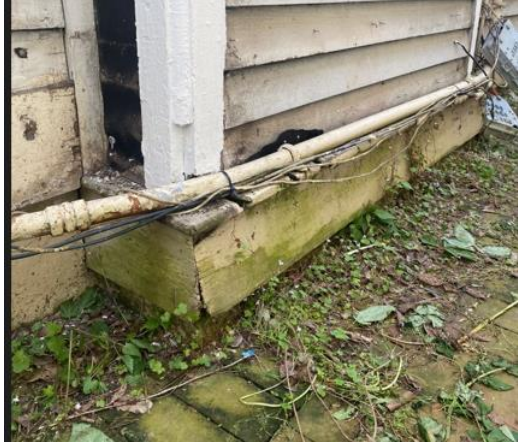
10: Old porch closed in to become living space. Poor condition
