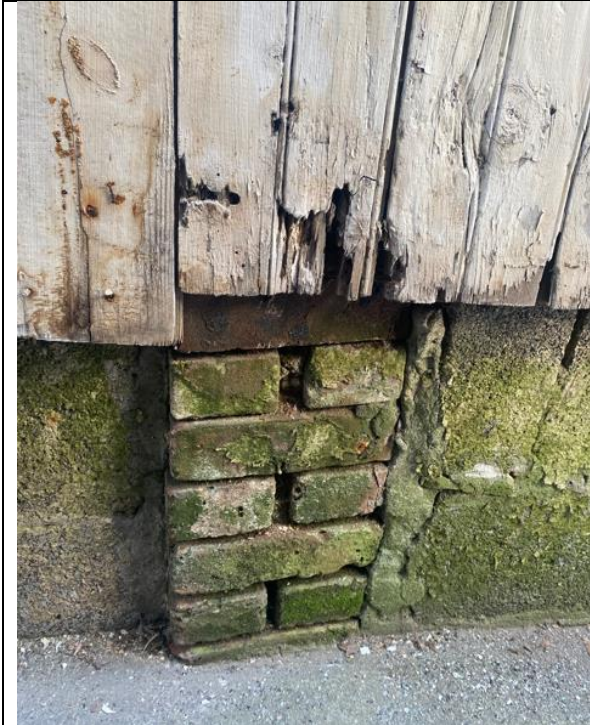
15: beadboard siding at rear in very poor condition
