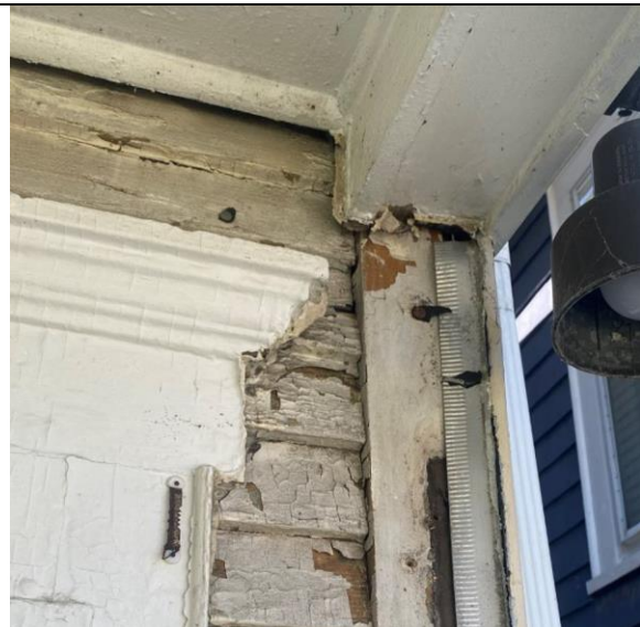
4: Evidence of rot and deterioration around the porch framing and corner of the structure on the first floor.
