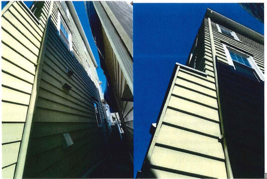
lower south wall of replaced clap; upper south wall with compromised clap
