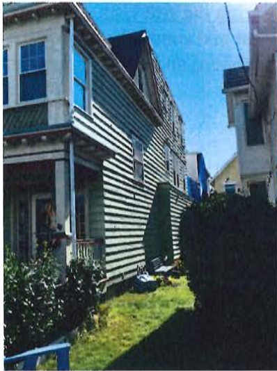
west elevation damaged clapboard
